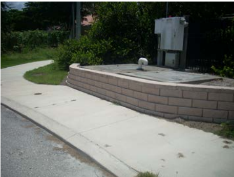
Hourly Rate for retaining wall repair: $_____ /hr Retaining wall at easterly terminus of 3 rd Avenue North (same style wall also found at Diana Ave & 13 th St N)
